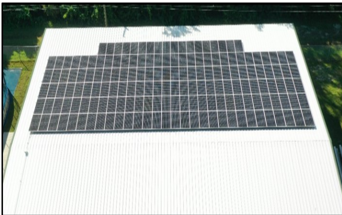
Solar Panels – Ruskin Recreation Center
